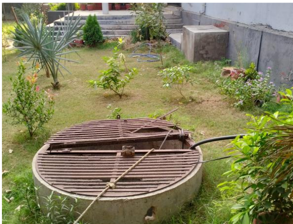
Rainwater harvesting well
